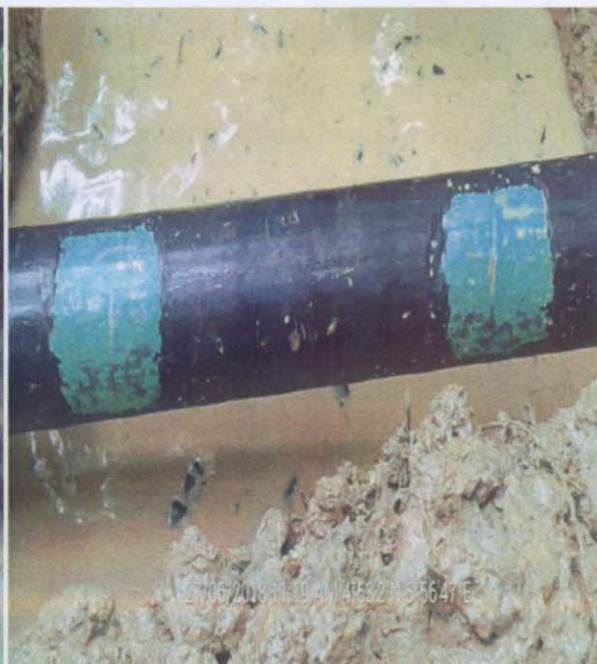
HACKSAW CUT ON FACILITY.
